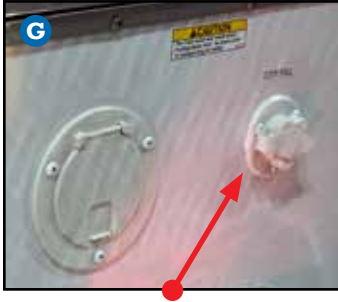
The city fill is located beneath the mechanical closet door side.
