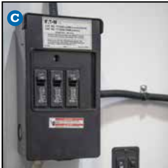
Electrical Panel Box
