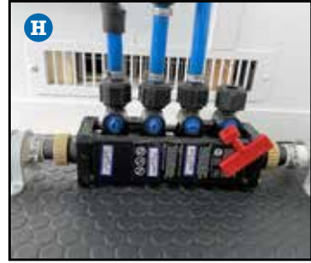
The Water Flow Control Center (main manifold) is where operator will adjust setting for City Fill or On-Board Water Supply
